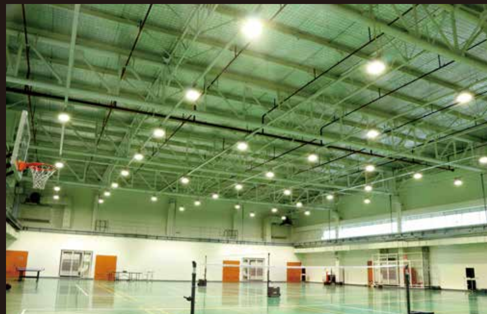
Lights for the gym in Asian Stanley, Thailand
